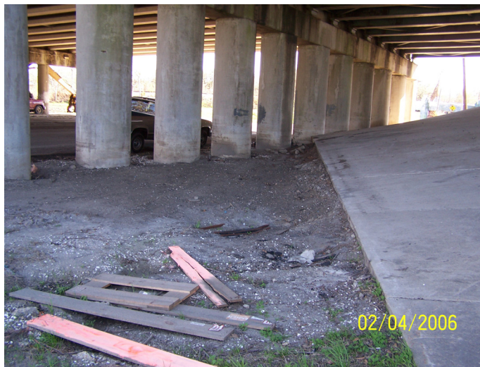
Figure 51. Erosion around the support structures for I-610 near Orleans Canal on Marconi Ave (Stop 6).
