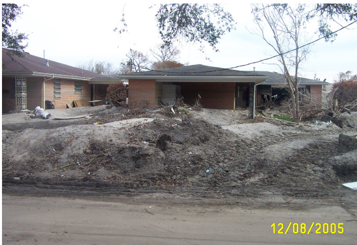
Figure 38. Sand deposits in front of houses on Pratt Drive at the North breach of the London Ave. Canal.
