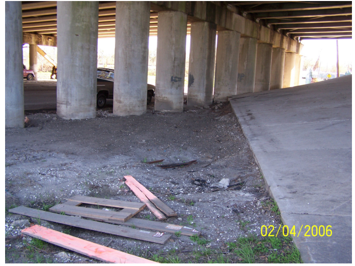
Figure 41. Erosion around the support structures for I-610 near Orleans Canal on Marconi Ave.
