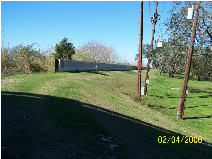
Figure 40. End of floodwall on Orleans Canal just north of I-610 overpass near Marconi Ave.
