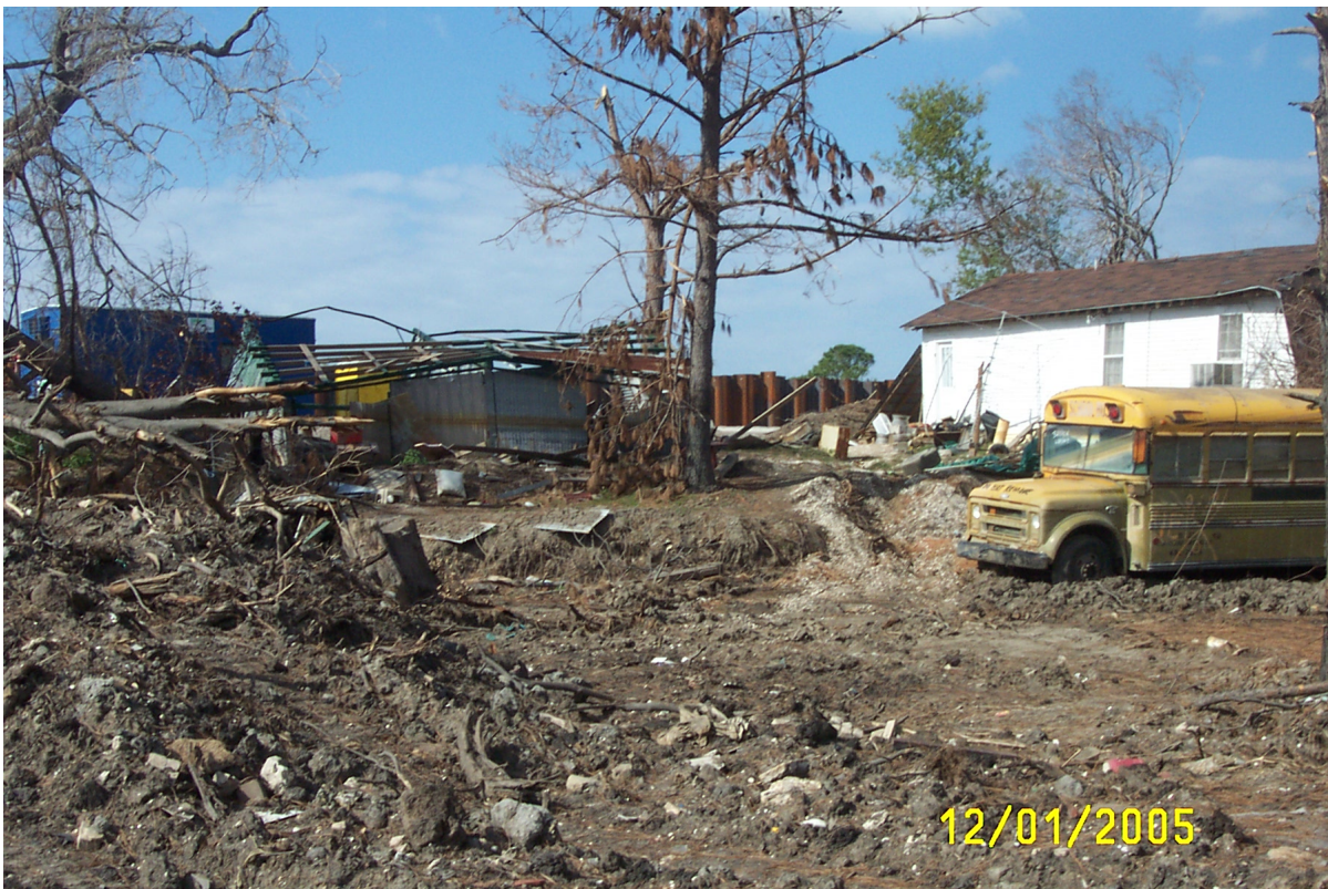
Figure 33. Slide toe (at abrupt change in slope in front of school bus) where levee and neighborhood were displaced about 45 feet toward the viewer.
