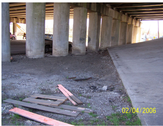
Figure 41. Erosion around the support structures for I-610 near Orleans Canal on Marconi Ave.
