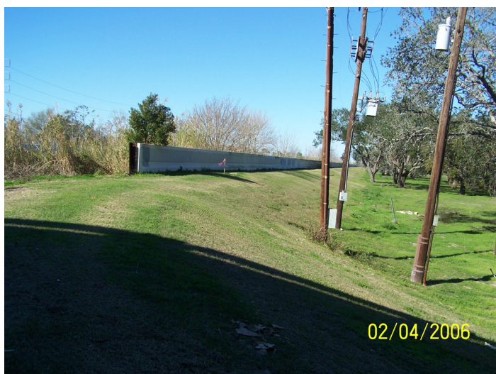
Figure 40. End of floodwall on Orleans Canal just north of I-610 overpass near Marconi Ave.
