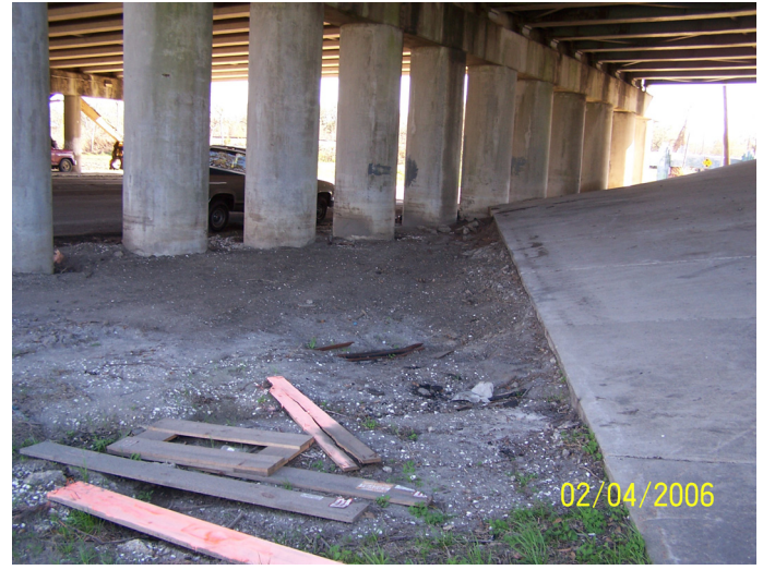
Figure 51. Erosion around the support structures for I-610 near Orleans Canal on Marconi Ave (Stop 6).
