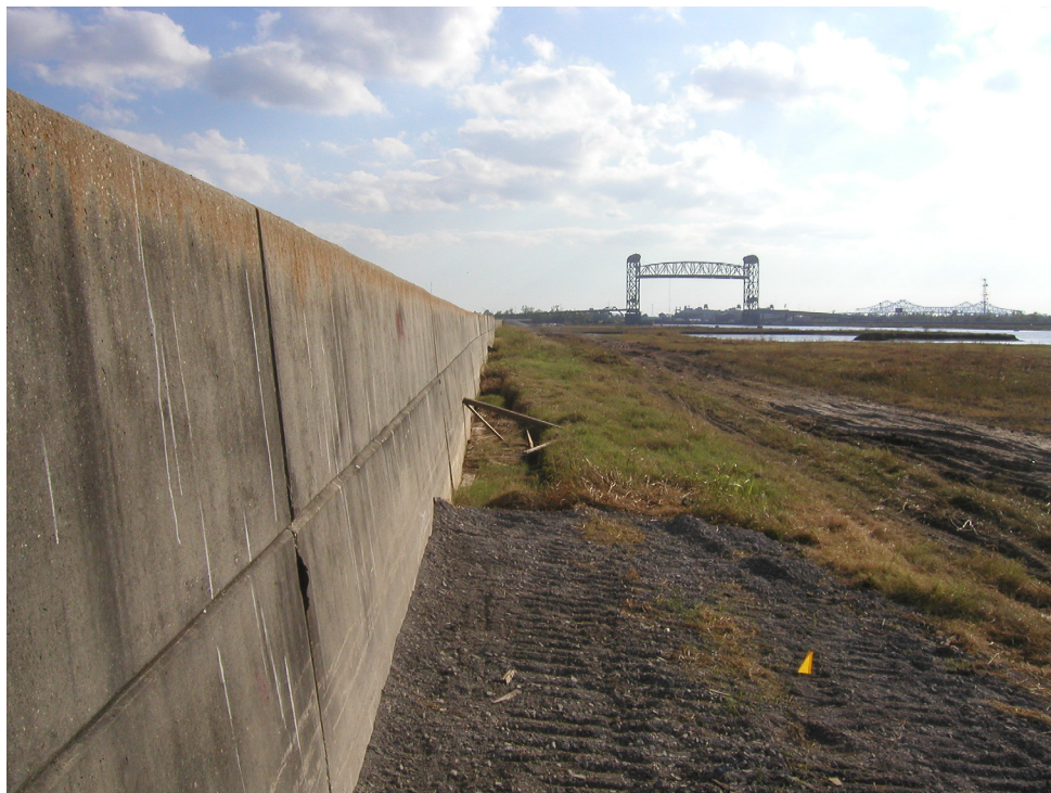
Figure 18. Looking South along the floodwall of the Industrial Canal on the inside of the floodwall between the two breaches showing the floodwall leaning toward the left (east) with a block of the levee next to the floodwall dropped down (near center of picture). Claiborne Ave. Bridge in right center. Photo from U.S. Army Corps of Engineers IPET web site, taken October 4, 2005.
