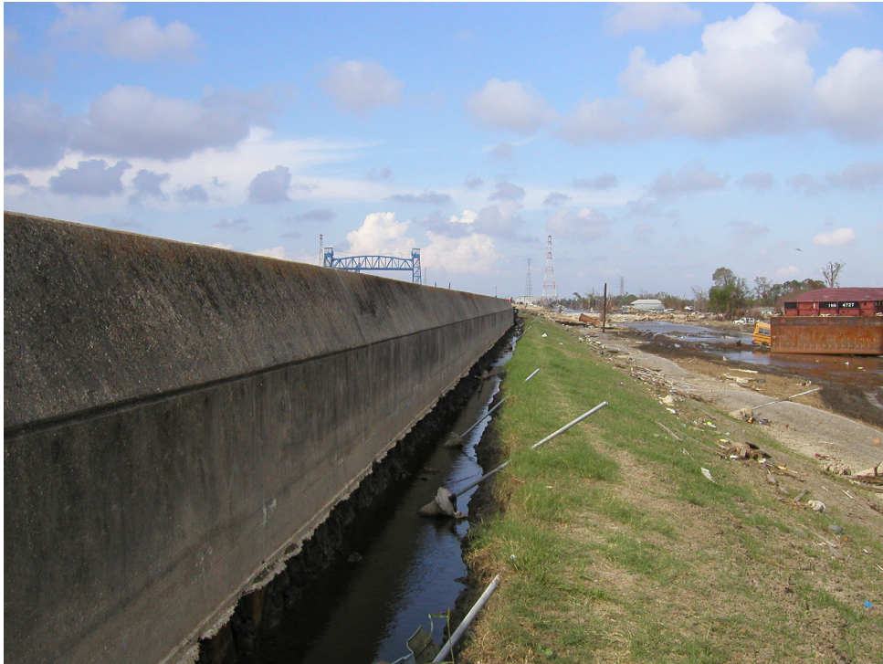
Figure 17. Looking North along the floodwall of the Industrial Canal levee showing trenches eroded by water from the Industrial Canal that overtopped the floodwall. Breached section is just beyond the barge and barely discernable in this view. Florida Avenue Bridge (blue) in upper center. Photo from U.S. Army Corps of Engineers IPET web site, taken October 4, 2005.
