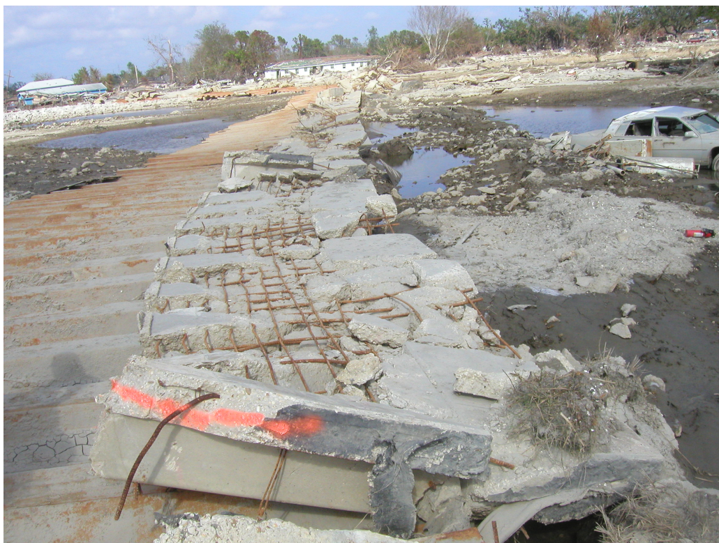
Figure 15. Floodwall and sheet piling strewn into Lower 9 th Ward at the southern (larger) breach on the Industrial Canal. Photo from U.S. Army Corps of Engineers IPET web site, taken October 4, 2005.
