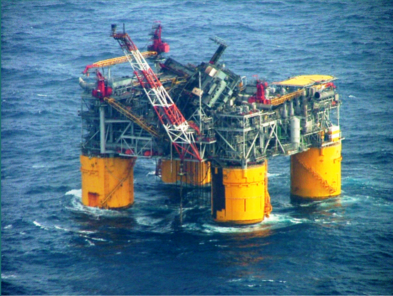
Platform Rig Derrick Collapse – Hurricane Katrina
