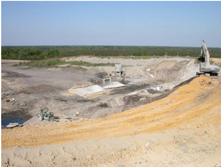
A view of the Woodside Landfill in Livingston Parish operated by Waste Management of Louisiana, LLC
